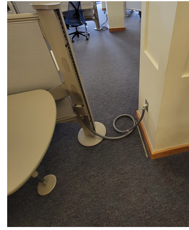
TYPICAL HARDWIRED FURNITURE WHIP CONNECTION (SHOWN IN ITS CURRENT LEVEL 3 LOCATION). TO BE RELOCATED TO LEVEL 1 AND RE-POWERED AS NOTED.
