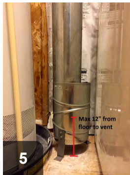
5 Terminate low vent within 12" of the floor. This one is fastened to a section of larger diameter duct for stability
