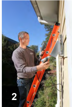
Test flue gases for carbon monoxide at outlet of vent
