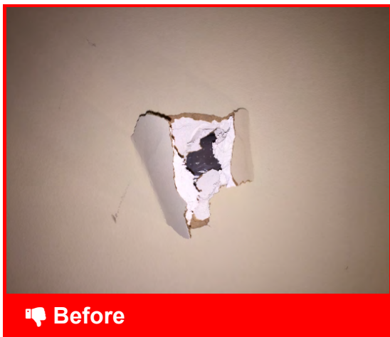
Replace any missing insulation and repair holes in vapor barrier
