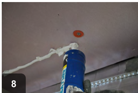
8 When insulating around low-hanging ducts and water pipes, run a line of sealant before placing insulation
