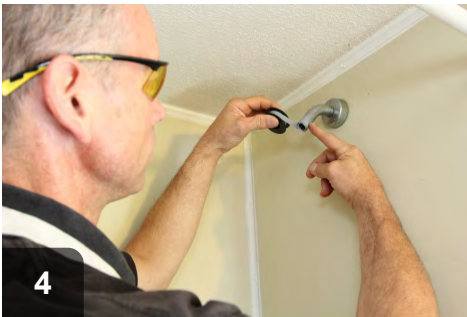
4 Seal the threads on the shower nipple with two wraps of Teflon tape. Wrap tape clockwise so it won't peel off
