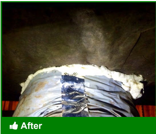
Crossover duct with vapor barrier mended and sealed to manufactured home belly
