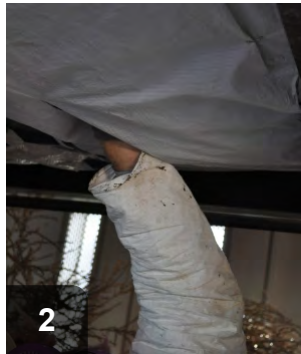
Holes in belly air barriers allow vermin access to insulation and ducting
