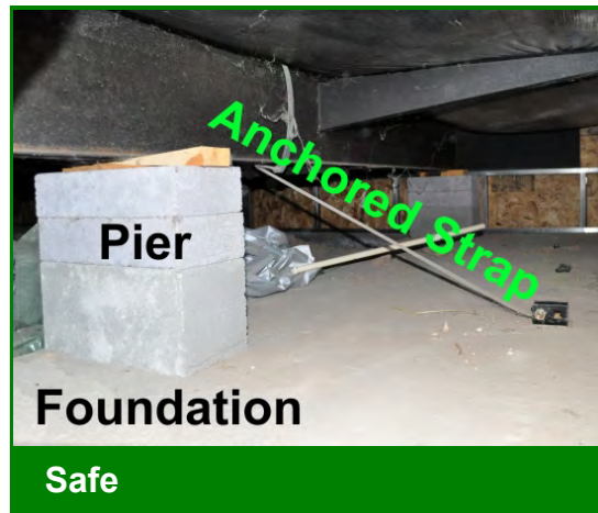
Safe Properly stabilized homes have a solid foundation and have anchored straps, unless otherwise indicated by manufacturer
