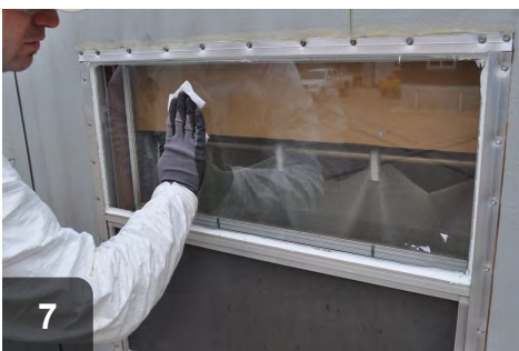
7 Clean glass to ensure than no out of place adhesive or glazing remains to bake onto glass
