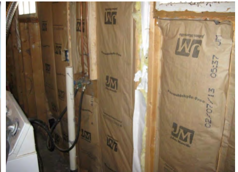
OR Kraft-faced fiberglass batts can be used with paper toward living space
