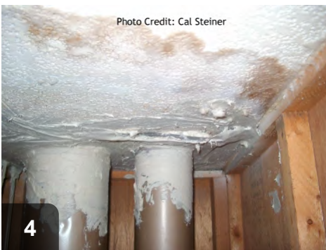
4 Photo Credit: Cal Steiner Inspect ceiling for weakness, leaks, clearance to combustibles, loose panels, and penetrations
