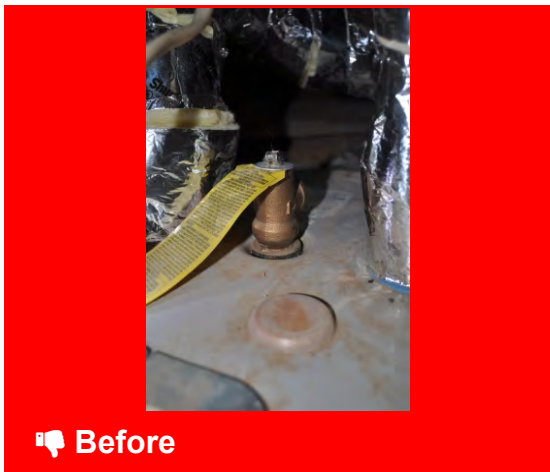
Water heaters should be not capped of at t&p valve
