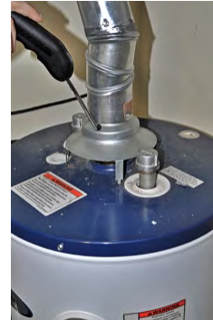
Test undiluted flue gases in natural draft water heaters
