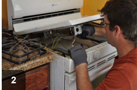
2 If CO issues are found, clean and tune appliances to remediate issues
