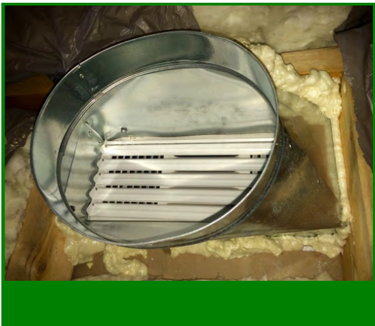
Register boot fastened to framing and sealed to gypsum with spray foam
