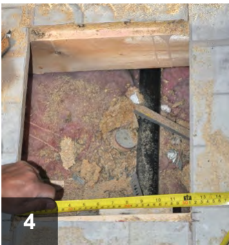
4 Once damaged area has been removed, measure for new patch and cut replacement subflooring to size
