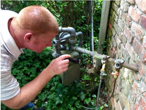
Inspect gas lines for corrosion, leaky fittings, worn flex lines, sediment traps and drip legs, and kinked copper
