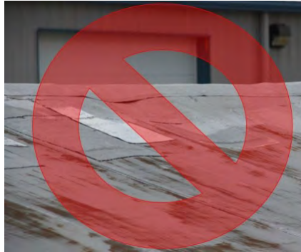
Dishing and pooling issues must be addressed.
