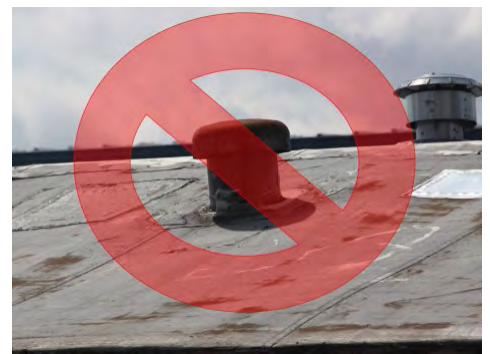
Mushroom vents must be replaced, or removed and sealed.
