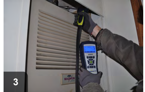
3 Test combustion appliances to ensure proper operation
