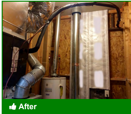
Additional combustion air supplied from high/low vents
