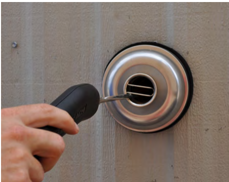
Test accessible exhaust outlets for power-vented appliances
