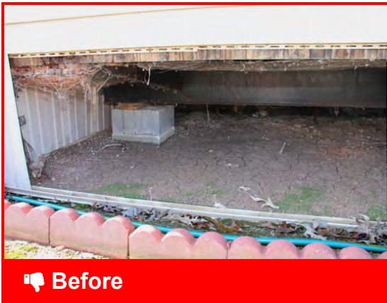
Manufactured home crawlspace with incomplete ground vapor barrier
