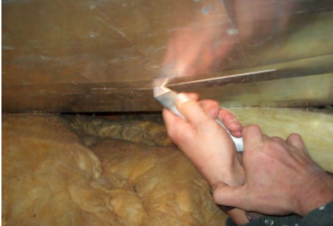
Cut belly to expose duct trunk. Use a utility knife to cut access under furnace plenum
