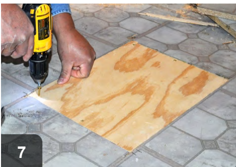
7 Securely fasten new subfloor in place, attaching to joist or blocking as necessary
