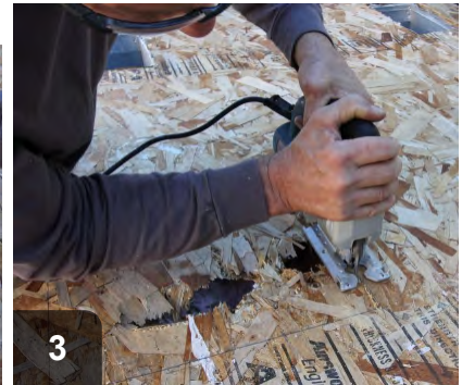
3 Cut out damaged area even with the inside edges of the floor joists
