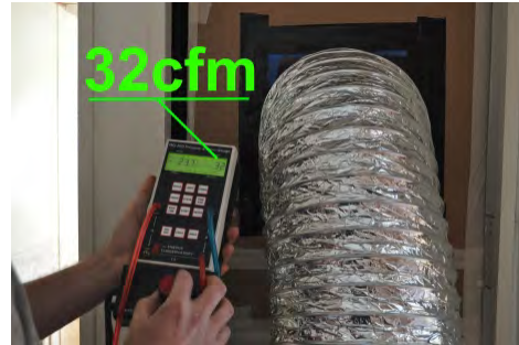
Perform duct blaster testing after completion of work and compare to 'before' reading. Record results
