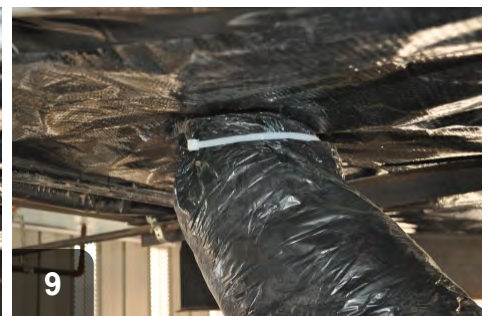
9 Use band tensioner to ensure that insulation and casing remain tight against belly
