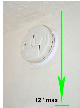
Wall mounted smoke alarms must be mounted within 12 inches of the ceiling and per manufacturer's specifications
