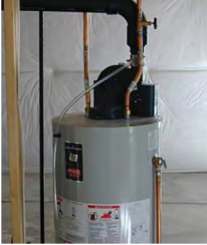
Power-vented water heater
