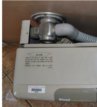
Ensure new combustion appliances are vented properly
