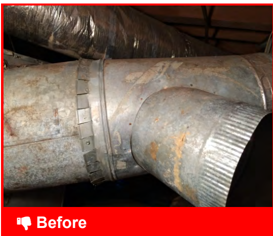
Unsealed metal ductwork
