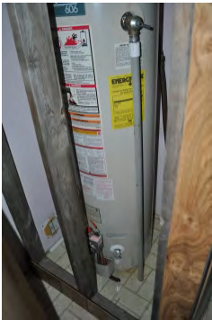
GOOD: T&P discharge should be piped within 6" of the floor or to outdoors
