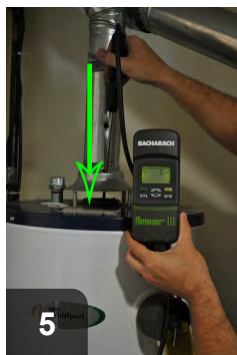
5 Check carbon monoxide levels on all combustion appliances
