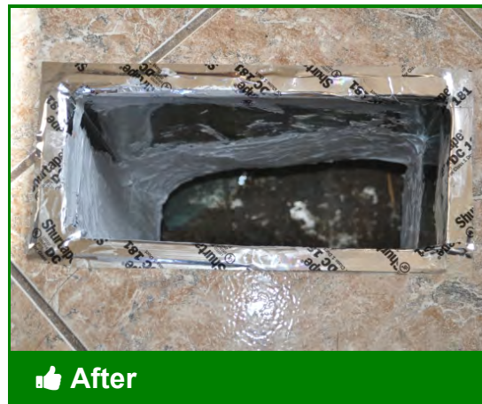
Damaged ducts should be repaired and securely fastened and sealed
