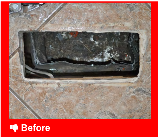
Unattached ducts are useless
