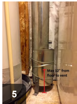
5 Terminate the low vent within 12" of the floor. This one is mounted inside a section of larger diameter metal duct
