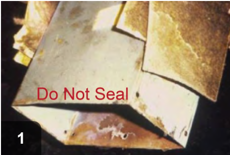
Label combustion air inlets with the words, "DO NOT SEAL"
