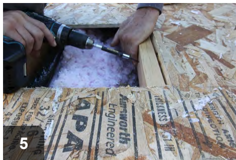
5 Install nailers flat against the joists. Finish by toenailing or screwing 2X4s between the joists
