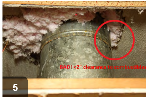
5 Verify at least 2" clearance to combustibles, unless flue is designed for zero clearance. Repair if needed
