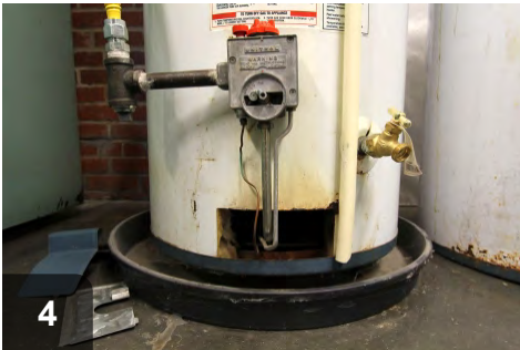
4 Inspect for signs of flame rollout, thermostat and gas valve condition, and proper T&P relief valve termination
