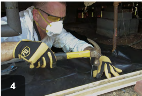
4 Secure vapor barrier to ground with corrosion-resistant landscape staples, or weigh it down with ballast
