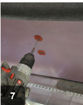
7 A rigid air barrier should be mechanically fastened to hold it tight against the floor joists
