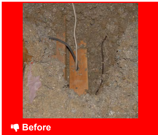
Unsealed penetrations through top plate
