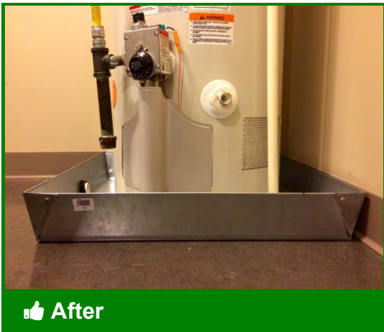
Emergency drain pan with drain piped to outside
