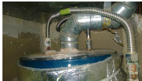
Inspect for missing draft diverter
