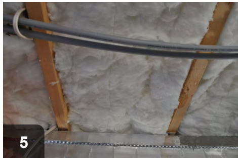
5 When ductwork or water pipes run below joists, insulation should be threaded above to fill joist cavity, uncompressed
