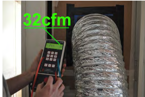
Run duct blaster test after work and compare with 'before' reading. Record result
