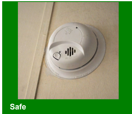
Hard-wired smoke alarm mount with alarm replaced
