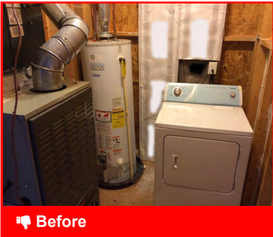
Combustion appliances in a confined space
