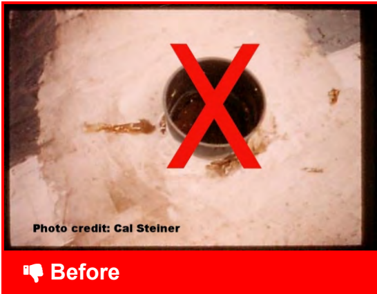
Roof leak, missing cap on vent
