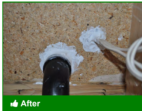
Gaps should be sealed to maintain air barrier
