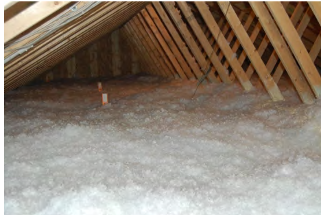
OR ducts can be buried in loose fill in attic spaces in drier climates
