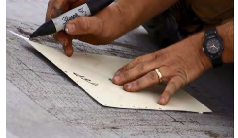
Use a 10"x10" sheet metal patch to mark the center of the hole.
