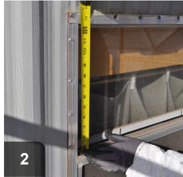
2 Measure sash for height of replacement glass -- cut glass to 1/4" less than sash height
