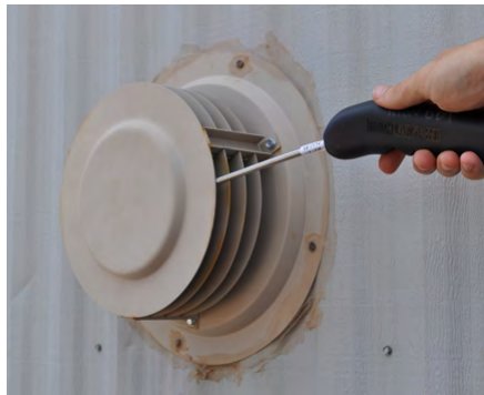
Test accessible exhaust outlets for direct-vent appliances
