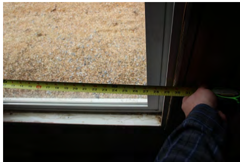
Windows are the proper width for egress.
