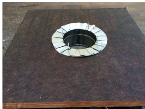
Starting collar with tabs bent over and screws through the duct board and backer ring
