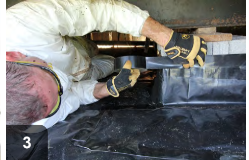
3 Wrap piers and columns at least six inches high. Use additional material to cover any gaps and holes in vapor barrier
