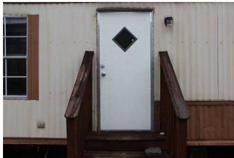
Manufactured housing should have two egress doors located away from one another. Stairs or ramps may be needed outside.
