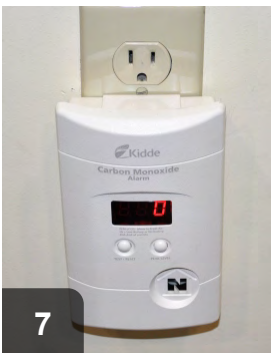
7 Verify safe levels on more than one instrument and in more than one location
