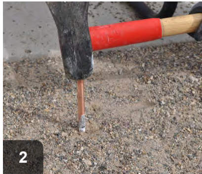
Grounding rod should be driven into the ground so that nearly all of rod is underground
