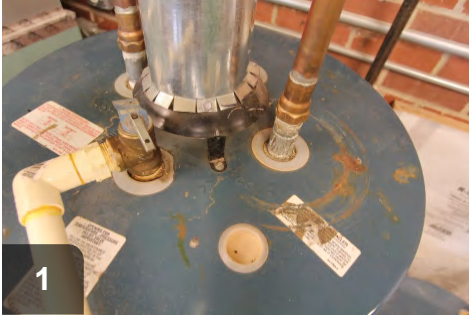
1 Inspect for rust, corrosion, and dust around draft diverter. Verify diverter is centered and fastened. Check T&P valve
