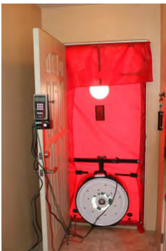
Set-up blower door to perform pressure pan testing before and after work
