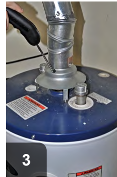
3 Test combustion appliances to ensure proper operation
