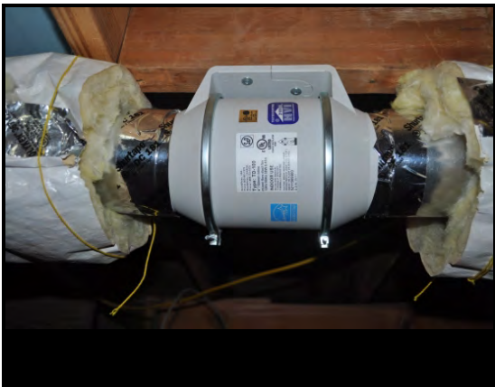
Appliance exhaust, such as that for a dryer, can cause depressurization
