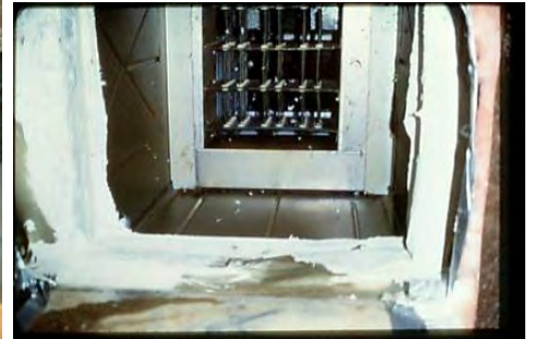
Using mastic and mesh tape, fully seal the furnace to the trunk line. Repair and seal the access holes in duct and belly
