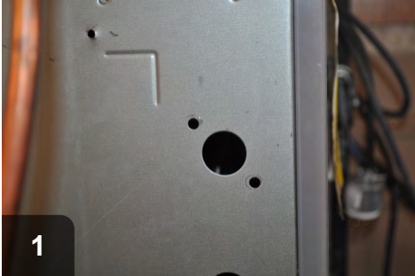
1 Unnecessary holes in the air handler cabinet should be sealed
