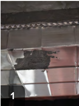
Holes in ducting should be patched to discourage vermin
