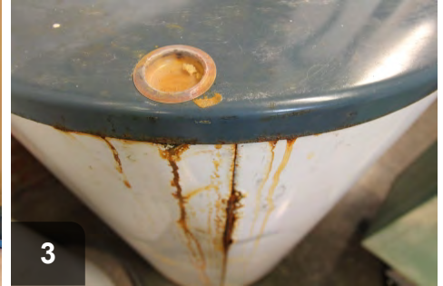
3 Inspect for rust, corrosion, and leaks
