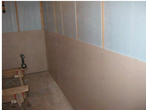
The drywall still provides an air barrier to keep moisture build up on wall
