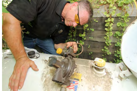
Inspect LP gas tanks for corrosion, proper location, leaky fittings, and kinked or damaged copper
