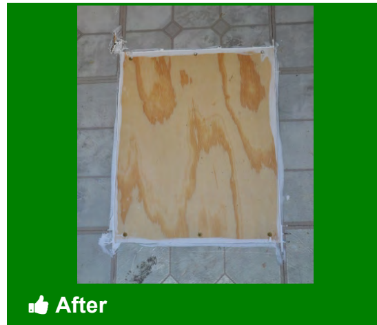
Completed floor patches should be air sealed to prevent leakage from belly
