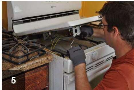
5 Appliance maintenance and air sealing are two ways to remediate CO leakage
