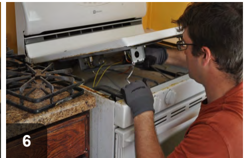
6 Appliance maintenance and air sealing are two ways to remediate CO leakage
