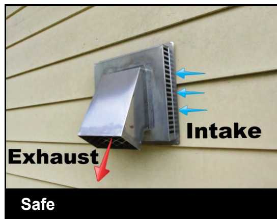
On-demand water heater combustion air intake and exhaust vent
