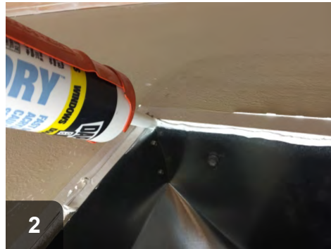
Caulk the boot to the gypsum board. Angle the tip forward and force caulk into the joint
