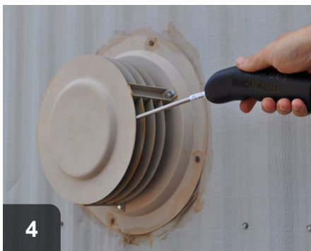
4 Check carbon monoxide levels on all combustion appliances, including direct vent equipment
