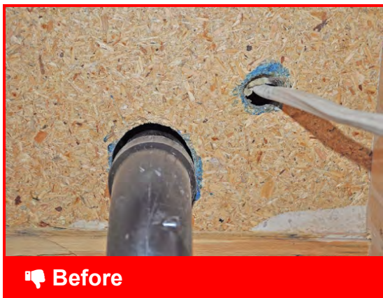
Gaps around floor penetrations, such as plumbing, HVAC, and electrical
