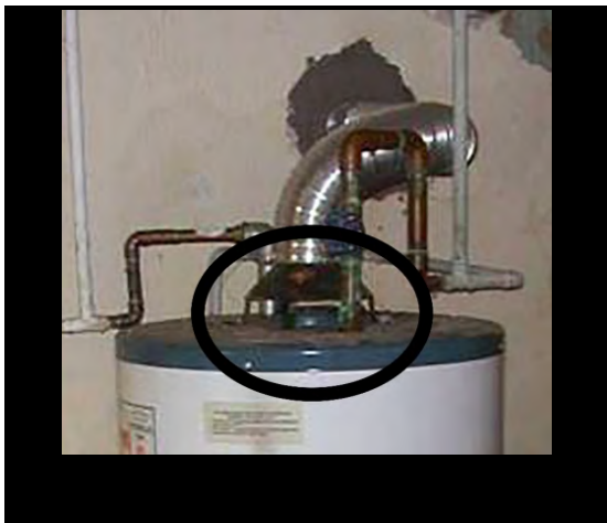
A natural draft water heater with draft hood highlighted
