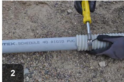
Attach grounding wire to fill tubes to minimize shock risk
