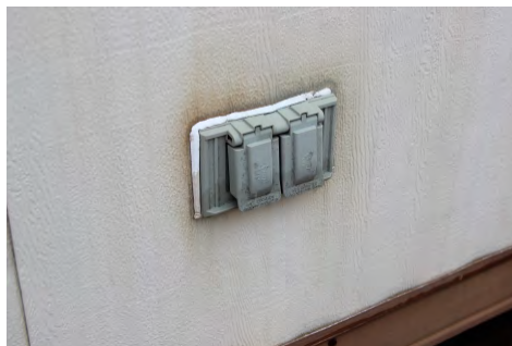
Exterior electrical outlet sealing.
