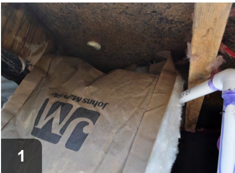
1 If fiberglass insulation is kraft-faced, ensure kraft is in contact with subfloor
