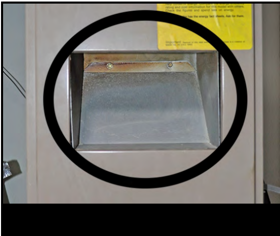
Category I 70% efficiency gas furnace with draft hood highlighted
