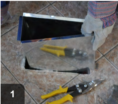
Replace damaged ducting if necessary
