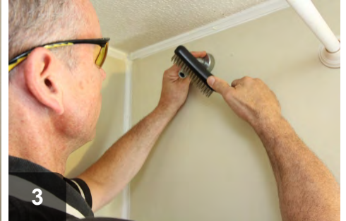
3 Clean corrosion and old sealant from the threads on the shower nipple using a wire brush
