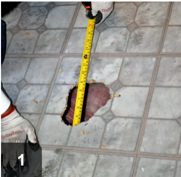
1 When possible, measure patch to reach surrounding joist. If not, blocking will be required.
