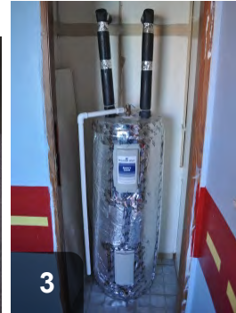
3 Adjust water heater settings and insulate as needed
