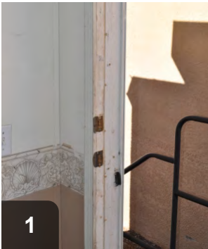
1 Door jamb is missing any weatherstripping
