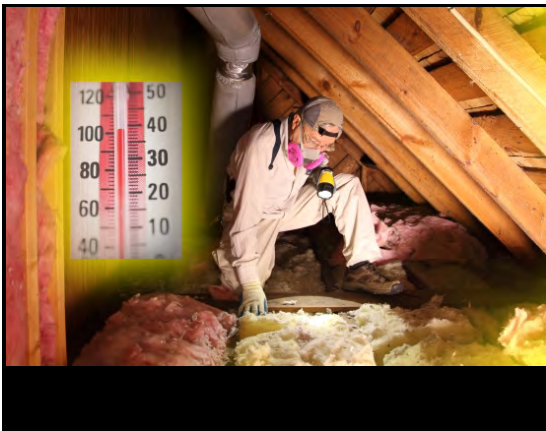
Attics and crawl spaces can be dangerous work places in the heat
