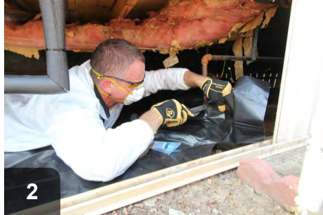
2 Measure, cut, and spread vapor barrier material after removing debris over 1/2" in size. Notch around obstructions
