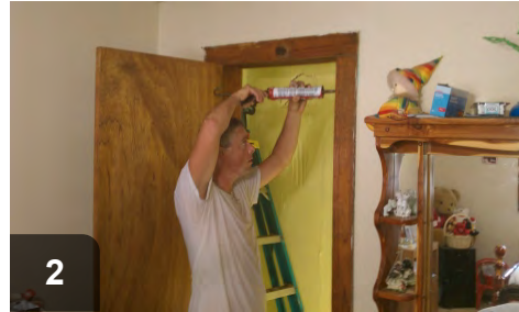
Foam, caulk, and seal leaks between halves of double wide manufactured homes
