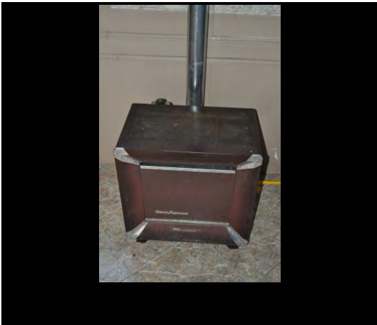
Natural draft appliances should be tested for spillage
