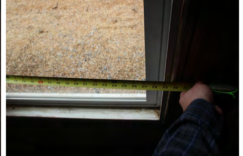
Egress windows should be more than 20" wide.
