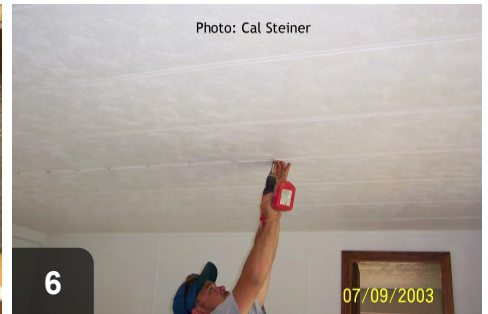
6 Photo: Cal Steiner Repair and refasten sagging or unsecured ceiling panels. Caulk and seal seams to prevent insulation spilling into house
