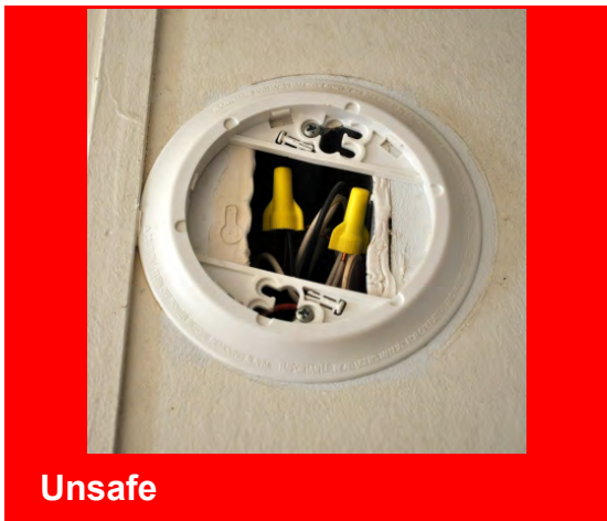
Hard-wired smoke alarm mount with alarm missing
