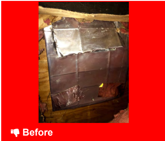
Access hole cut into manufactured home branch duct
