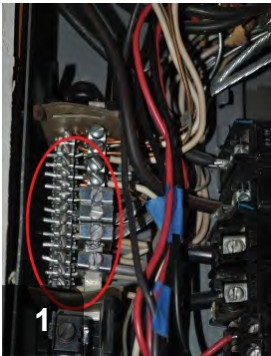
Inspect panel box for presence of (silver or gray colored) aluminum wire
