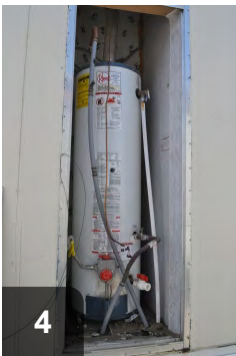
4 In older mobile homes, the water heater closet may be accessed from the exterior
