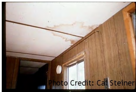
Inspect ceiling for weakness, leaks, clearance to combustibles, loose panels, and penetrations.
