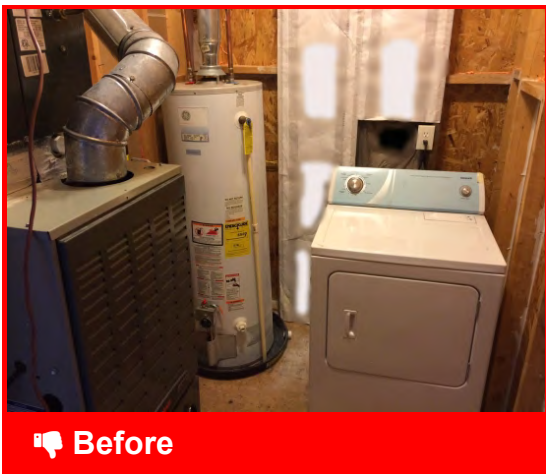
Combustion appliances in a confined space
