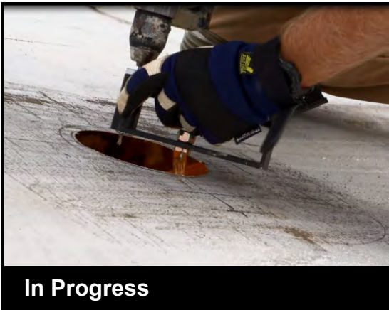
Rough cut hole that will need to be sealed.
