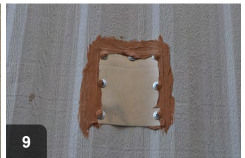
Securely fasten patch in place with screws and apply addition sealant to deter water
