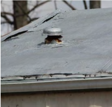
Plumbing stacks must be terminated to the outdoors.
