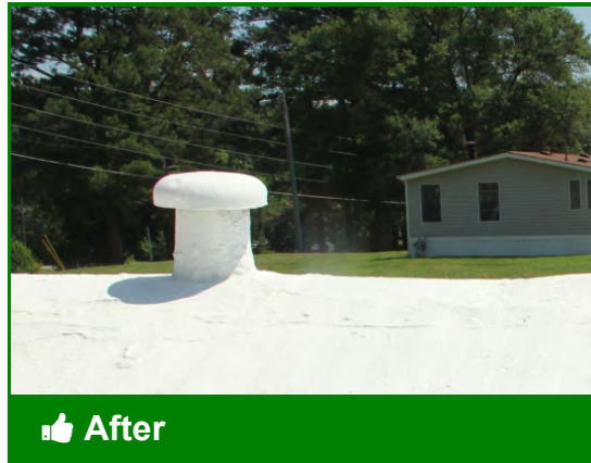
Properly connected and sealed roof vent
