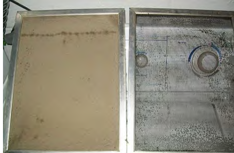
When a simple filter cleaning or replacement will help, make it happen
