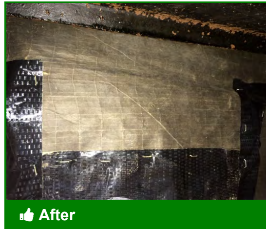
Repaired, insulated, and sealed access hole in manufactured home duct and belly
